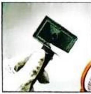
6: Once the seal is securely secured to the edge, glue the silicone seal along the edge of the gutter
