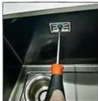
8: Use a power screwdriver to fasten wicker screws to the edges to reinforce the drain.
